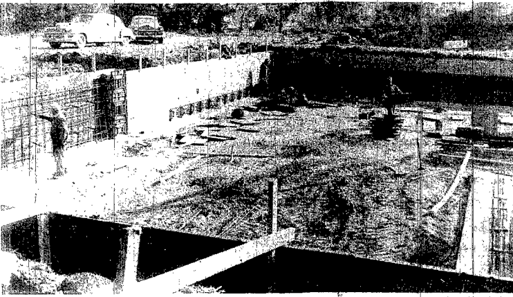
Work on Wayne's new swimming pool was moving rapidly this week as construction workers poured concrete for walls of the pool. The photo above shows the diving area and part of the main pool after first pours were made last week.
